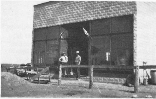
Installing gas pump at B. L. Smestad's new store. Notice the hitching posts!!
